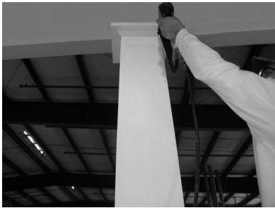
13) Apply glue to final 1/4 cap piece and biscuits and slide into place. Pin nail cap moldings to top of column.*
