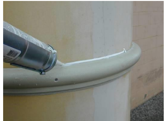
16) Apply a bead of good paintable exterior chalk at the top and bottom joint where the neck ring joins the column. Smooth bead for proper appearance.
