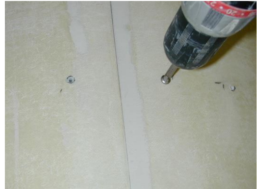
3) Reinstall pan head screws on the column half just assembled with adhesive.
